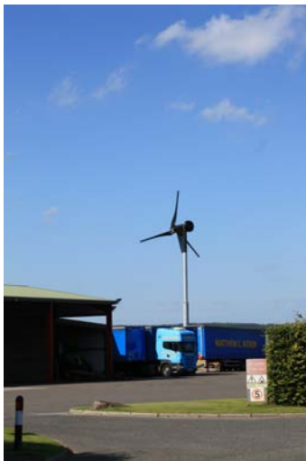
3 bladed Proven turbine on tubular tower
